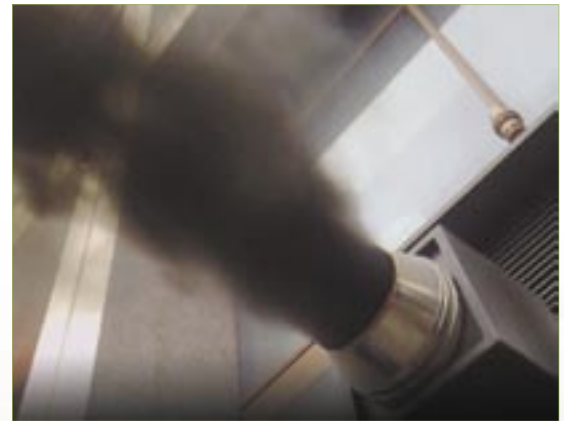
(Typical emissions from a standard diesel generator engine)
