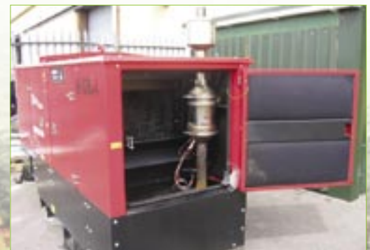
(Acti-Trap-F installed onto a mobile generator)
